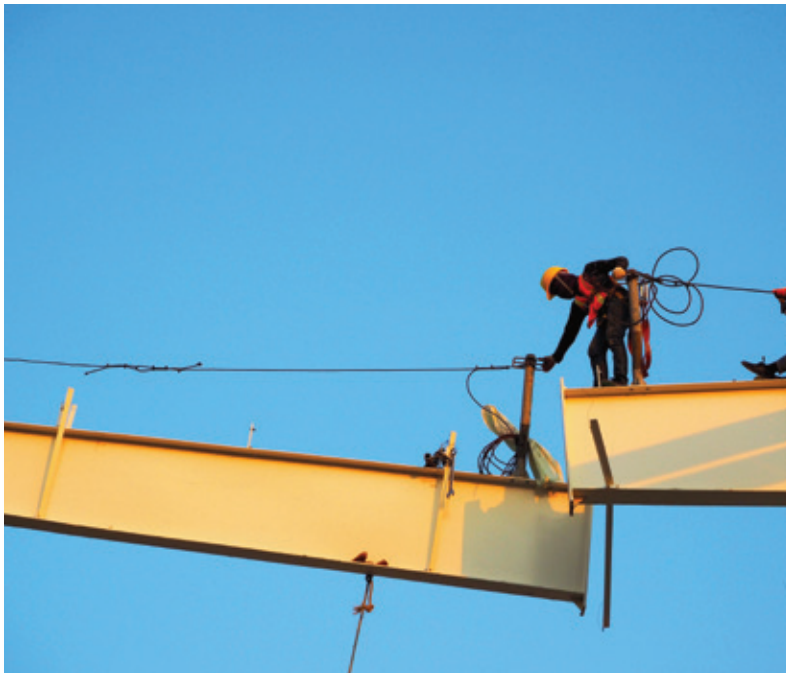
Working at height and in construction increases the risk for accidental falls.
