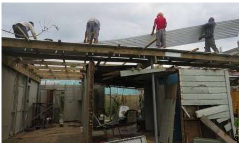
LEFT: The Tonga Leitis Association drop-in centre and office suffered heavy damage from tropical cyclone Gita. Rebuilding efforts were supported through the grant.
